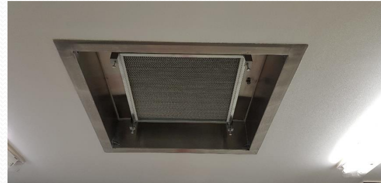
Clean room side of hepa module (shown without cover)
