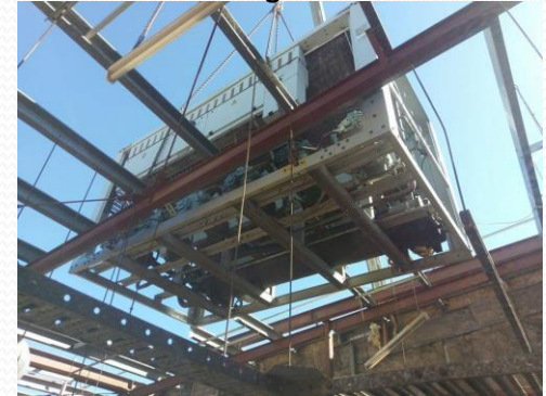
Anam Cara new Chiller in
