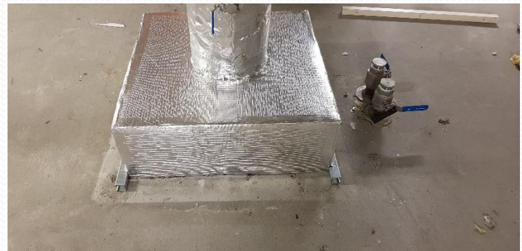
Plantroom side of hepa module
